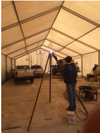
Building our well tripod. Top is separate so whole thing is transportable. It worked great!
