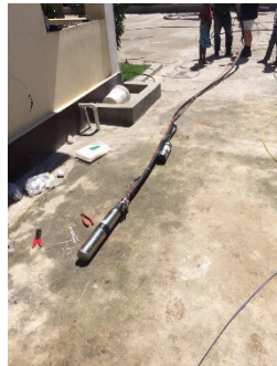
AC pump at bottom and DC pump above it
