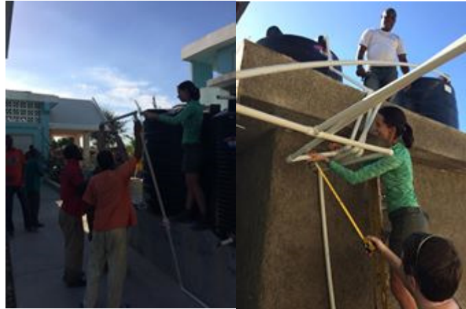
Plumbing in the pure water tanks Nic and Renee could do anything. up by the hospital – 100' from the They didn't teach PVC plumbing in engineering school though system
